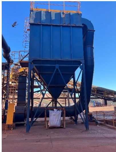
Dust Extraction System
