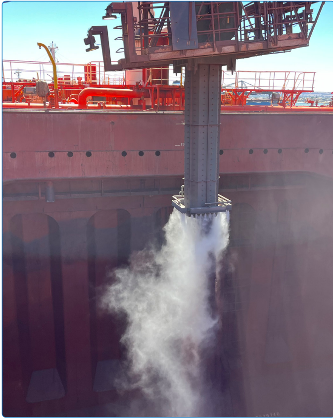
Berth 5 Shiploader Dust Suppression System
