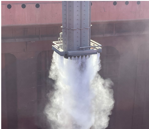
Berth 5 Shiploader Dry Fog System
