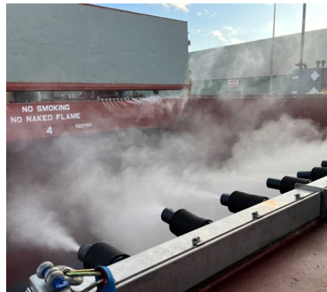
Berth 6 Vessel Hold Dry Fog System
