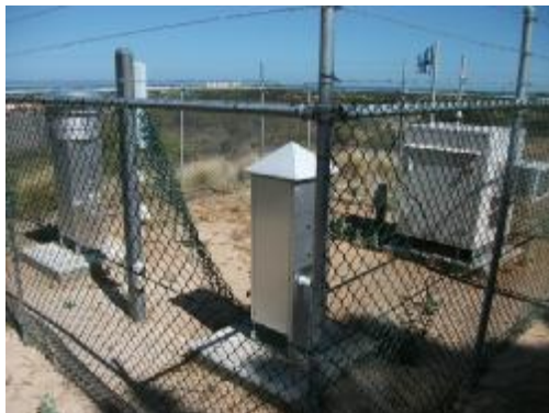
Figure 7 – Damage by vandals at Durlacher Street monitoring site
